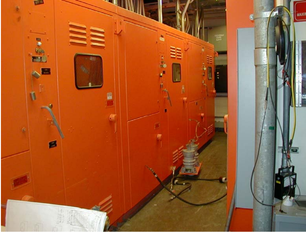
Figure 3, Safety Disconnect Switch Cabinets Containing Slow Bus Disconnects and Fast Ground Switches
