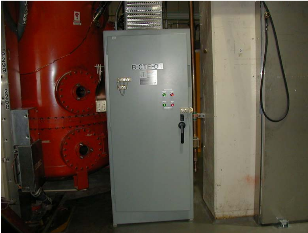
Figure 5 CTF Grounding and Disconnect Switch Enclosure
