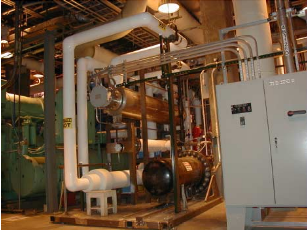
Figure 5-2 Similar Helium Bakeout System in Use on NSTX
