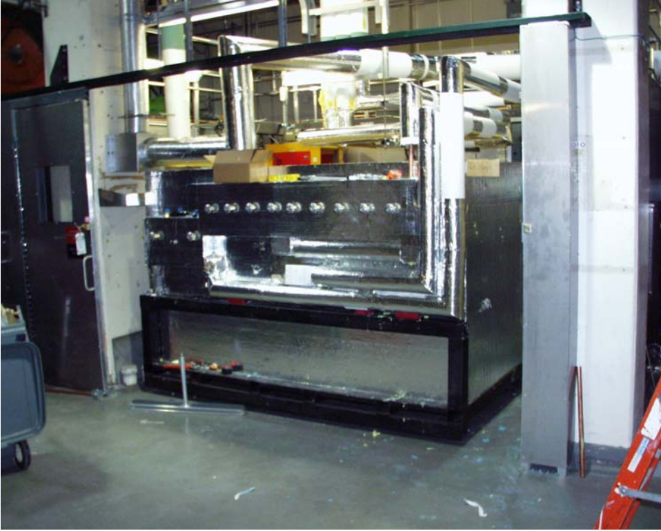
Figure 5-30 Cryostat inside Coil Test Facility
