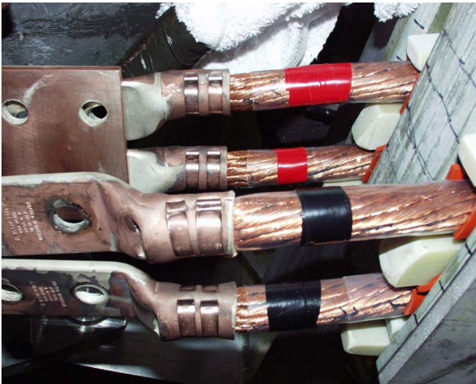
Figure 5-27 Crimped lugs on current feeds
