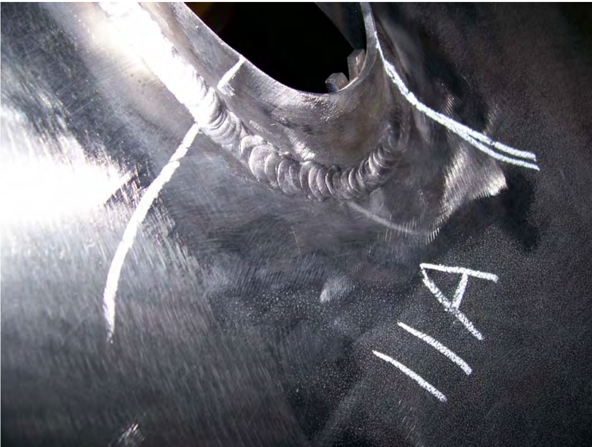
VVSA-1 Undersize fillet weld areas – port to vessel welds – 5/30/06
