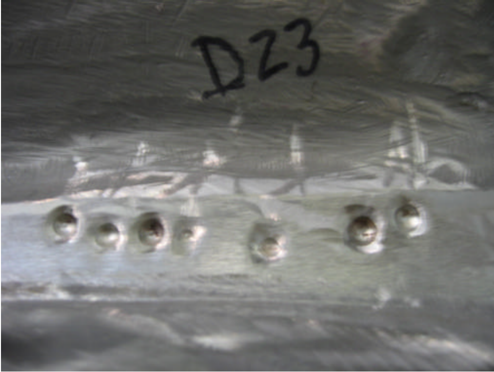
Excavated areas of high permeability beneath VPI groove in radius at casting wall.
