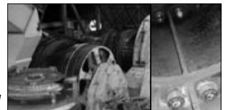
Hoist and drag drums.
