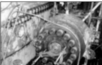
HP Turbine and valve
