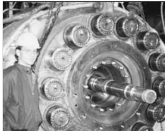
Ingersoll Rand boiler feed pump with 6" diameter studs (H650TX-600-8/w). With air tools, tightening required only 2-1/2 hours.
