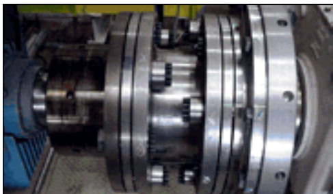
This flexible disc coupling took 2 men 2-1/2 hours to install, saving this company 19 man hours!
