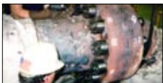
Steam turbine inlet flange. 30 minutes to install, 15 minutes to remove.
