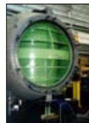
Split joint on new manufacture ball valve.
