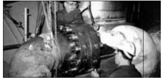
High pressure steam lead with rotational misalignment of bolt holes. Solved leakage and history of bolt failures.
