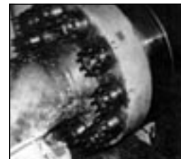
Excess let-down heat exchanger.
