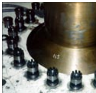
Radial expansion bolts used for generator rotor to shaft connection.
