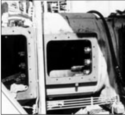
Reciprocating compressor, distance piece.
