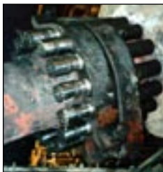
High pressure steam turbine inlet flange.
