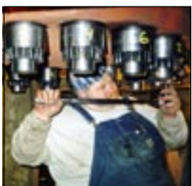
High pressure feedwater heater.
