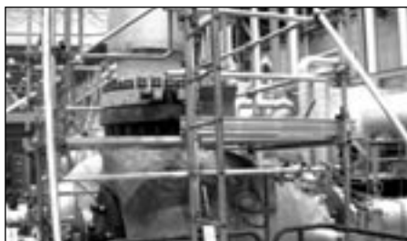
Steam inlet flange, control valve and stop valves on 960 MW turbine.
