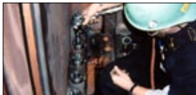
Stainless bolts used for blade rings and inner turbine shell.
