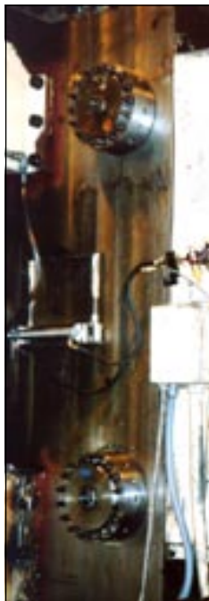
Superbolt Tensioners on a 1,000 Ton Diecast Machine.
