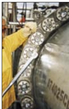
Final torque values on heat exchanger verified with hand held torque wrench.
