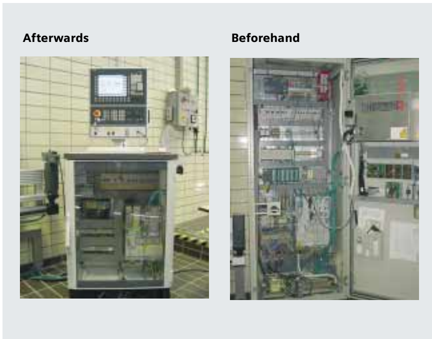
Fig. 10/6 Software replaces hardware components, electrical cabinets become smaller
