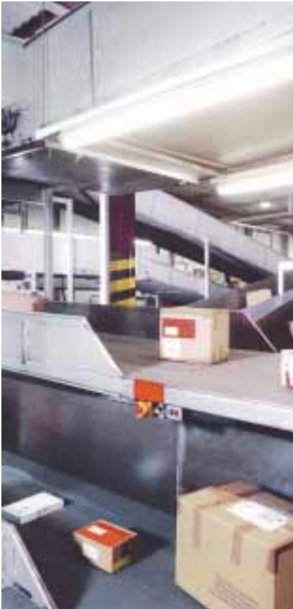
26 Siemens Emergency Stop command devices mounted at key locations in the parcel sorting system and connected with one another through AS-Interface
