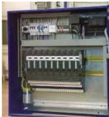
Fig. 5/6 Distributed electrical enclosure with ET 200S Safety Motor Starter Solution Local
