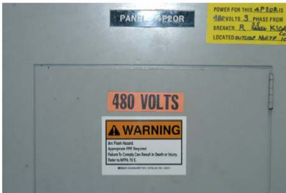
Figure 2-4. Warning label on Panel 4P20R
