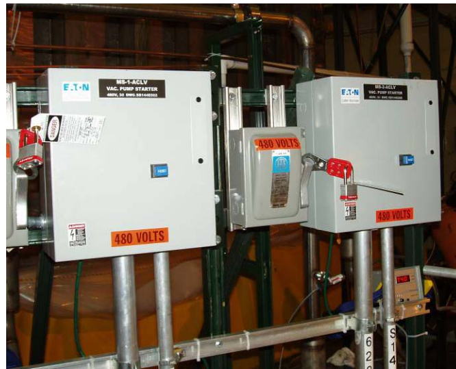
Figure 2- Vacuum Pump Starters
