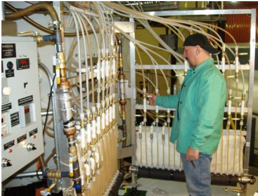
Epoxy Delivery Control Station
