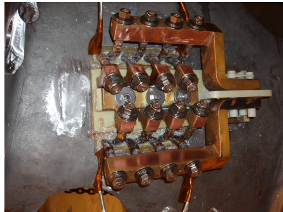
Modular Coil Lead Area
