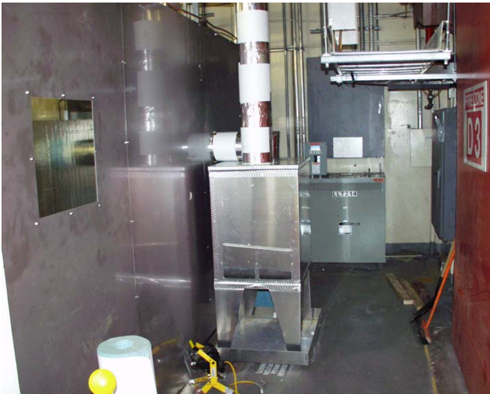
Figure 5-29 Connection of cryostat to facility exhaust
