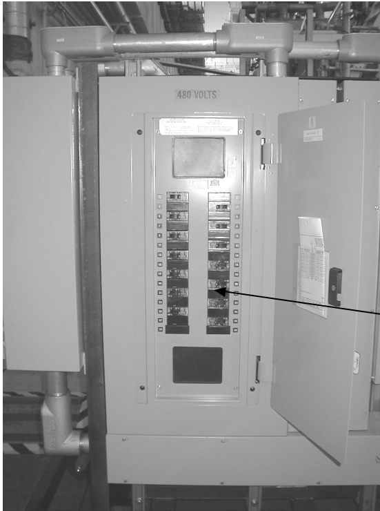
Figure 5: Chamber strip heater circuit breakers (Located near the south wall, on the power cart(s))
